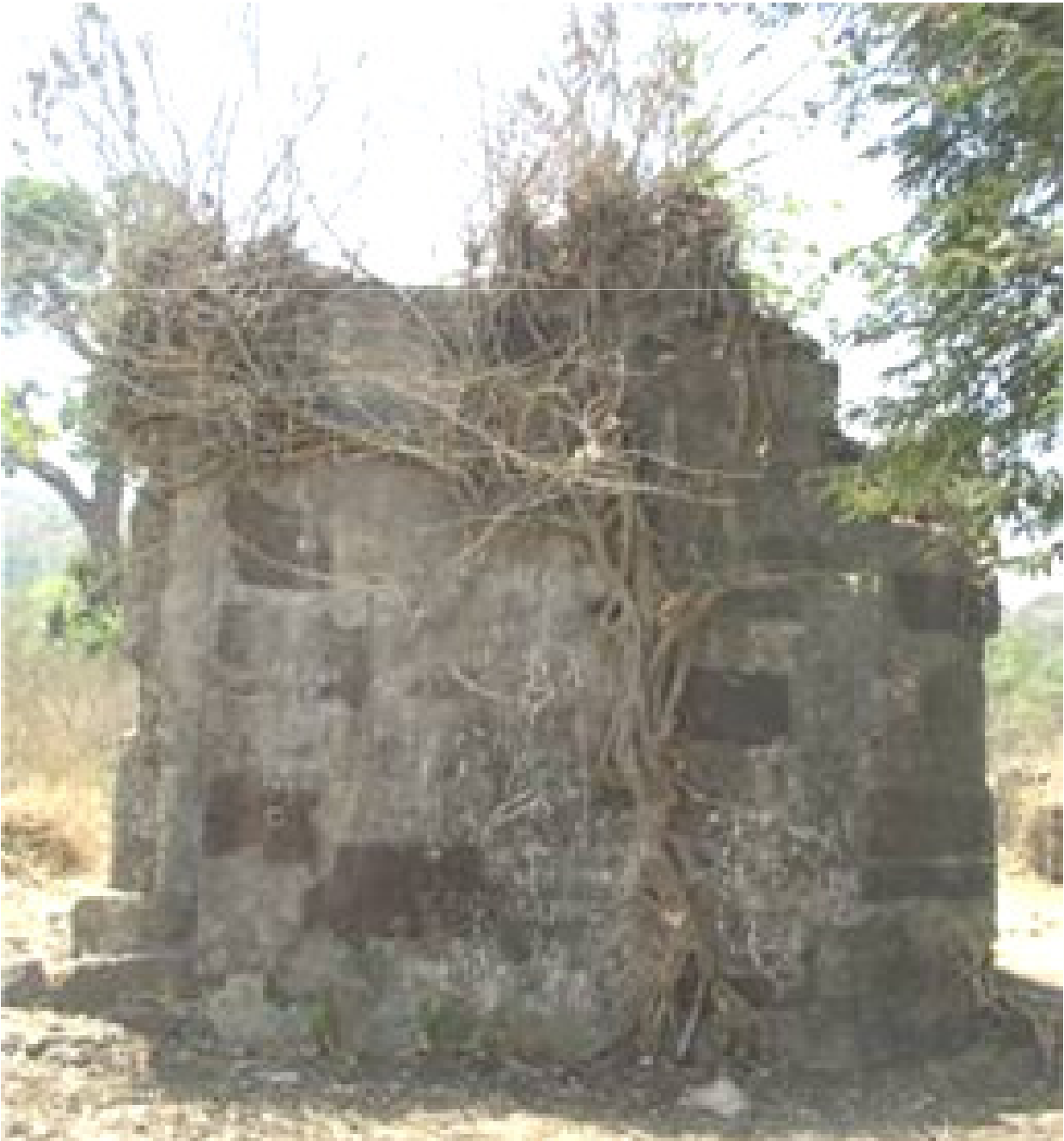
Derelict structure within the fort showing growth of vegetation
